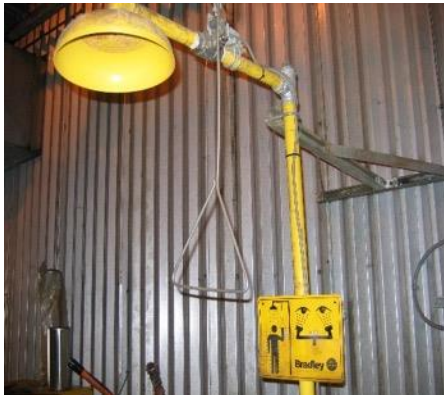
Plumbed-in safety shower
