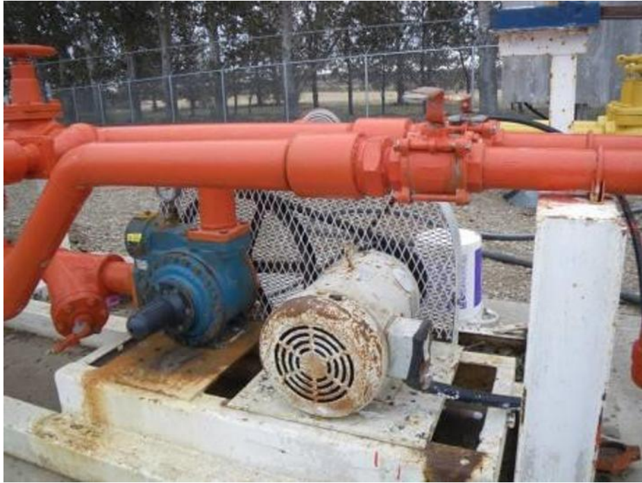
Figure 12. Guards on Transfer Pumps/Compressors – Example 1
