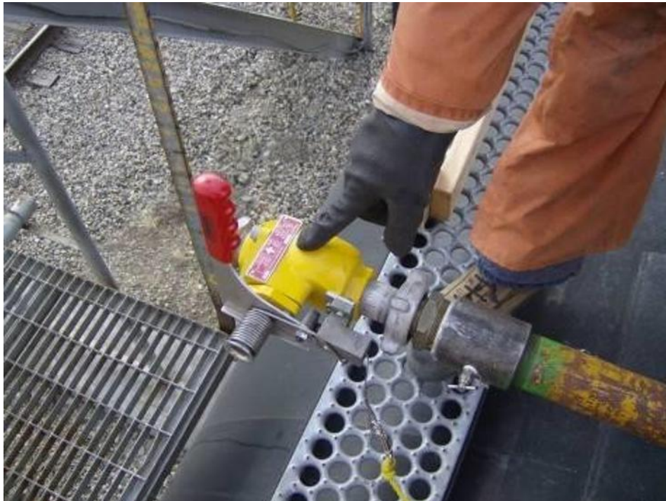
Figure 2. Emergency shut-off valve on a rail car.
