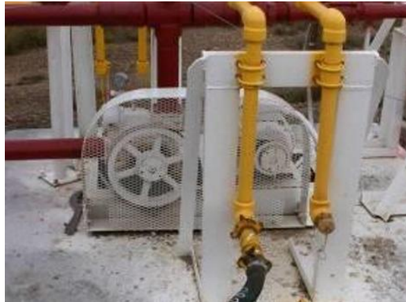
Figure 13. Guards on Transfer Pumps/Compressors – Example 2
